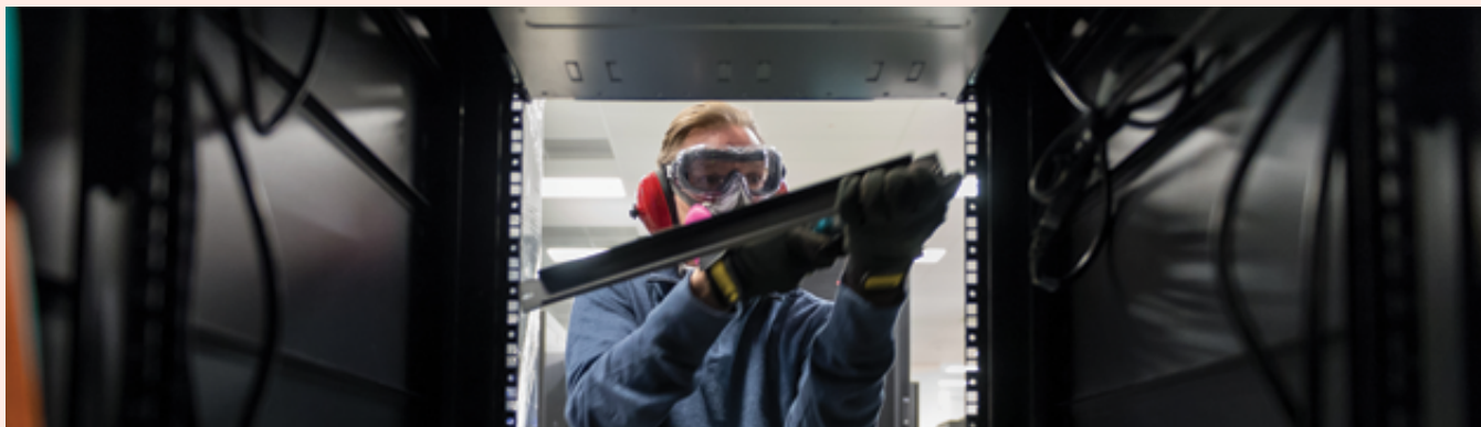
Ryan Milner, ALCF HPC systems and network administration lead, installs NVIDIA DGX A100 nodes as part of the Theta upgrade.
